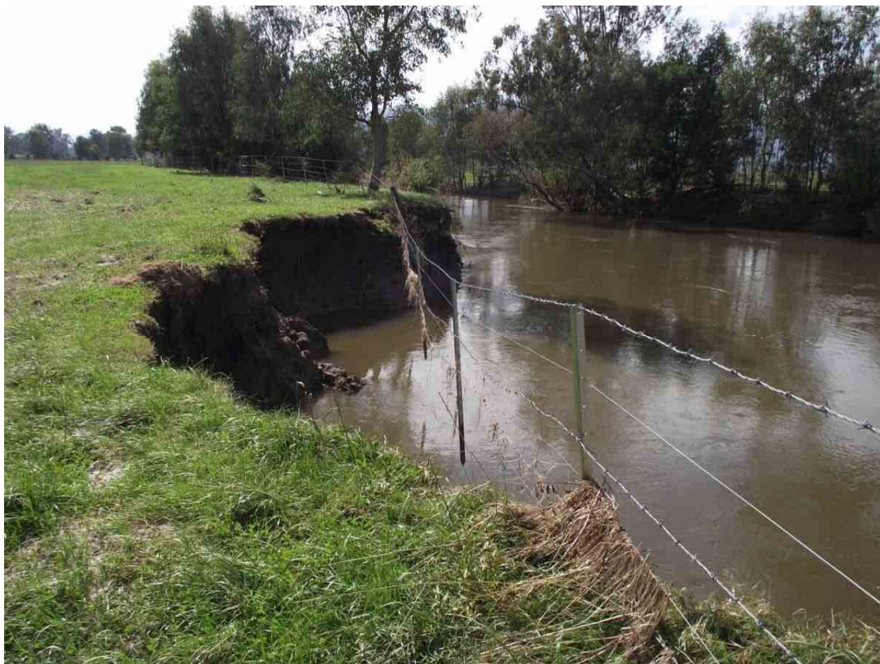
Figure 5.1 – What can happen to a riparian fence when it's located too close to the channel, Jeremal Creek (north-east Victoria) after the 2012 flood (photo: North East CMA)
